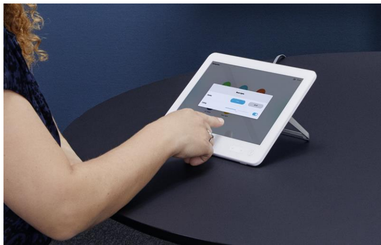
Figure 2. User interface displaying in-room control information
