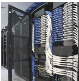
Figure 1. Production Data Center
